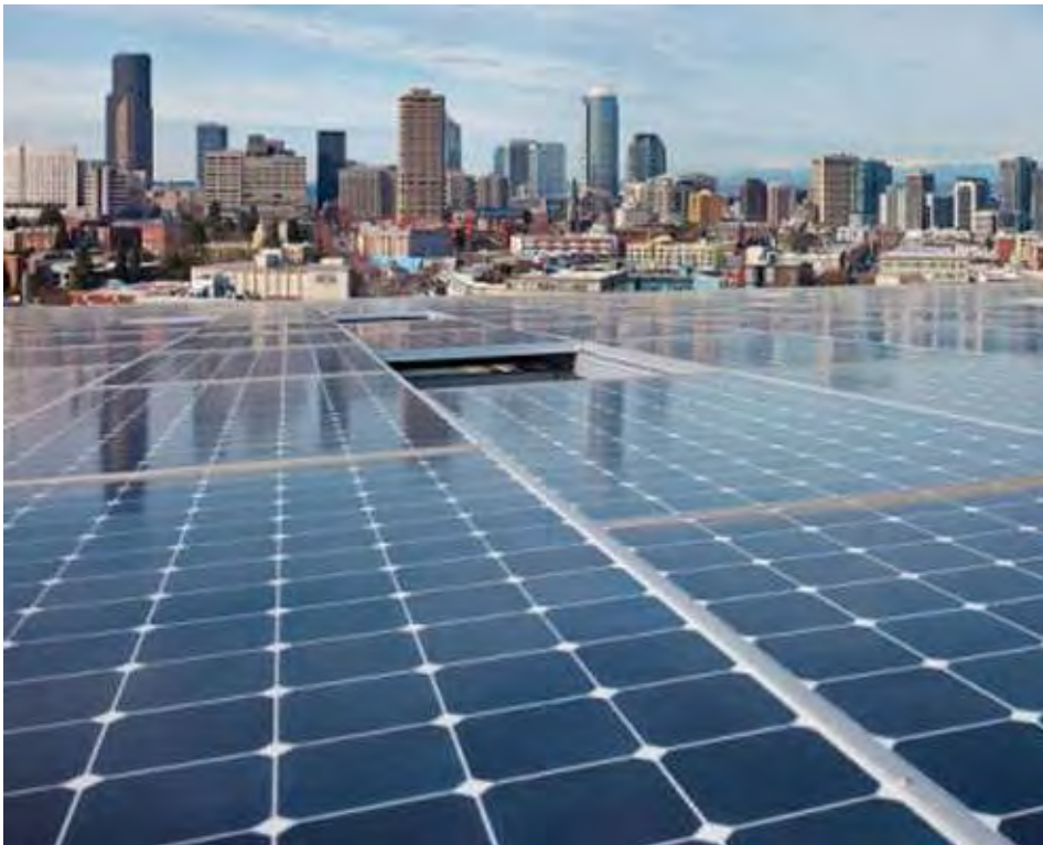
Figure 2. The Bullitt Center’s 242 KW PV (photovoltaic) array (Benjamin Benschneider).
